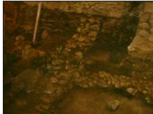
Figure.8:(b) An image showing foundation construction with rubble stone, Ahmed Katkhuda EL-Razaz (ARCE conservation project. Historical Cairo
