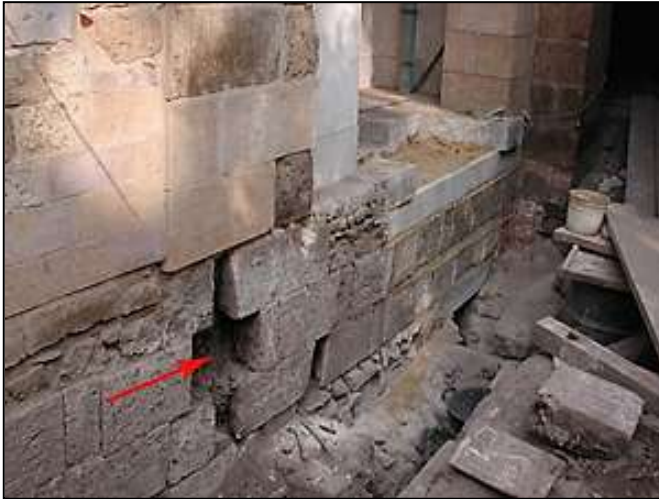
Figure. 11: (a) An image showing stones in a horizontal position. Ahmed Katkhoda EL-Razaz's house Foundations, Ottoman Era (ARCE conservation project)
